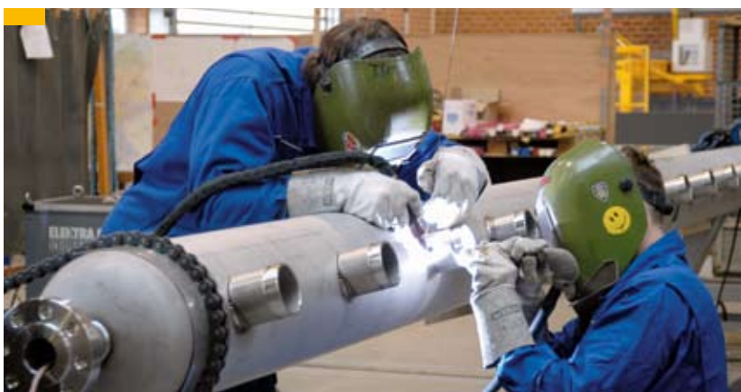
Fig. 33: Prefabrication of distribution pipes made from superduplex for a seawater desalination plant
