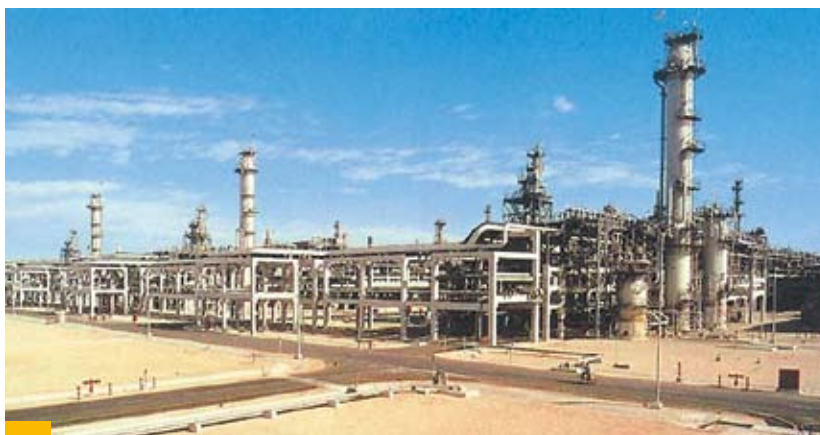
III. 31: Pipes for a desulphurization plant in Qatar
