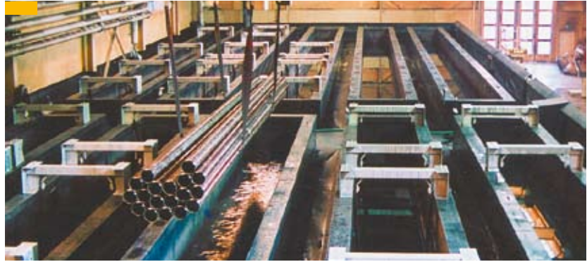
III. 27: Pipe pickling installation offering big capacities
