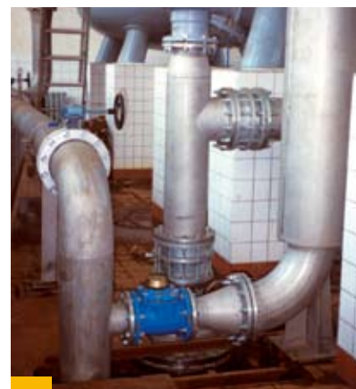
Assembly time can be drastically reduced with a high degree of prefabrication
