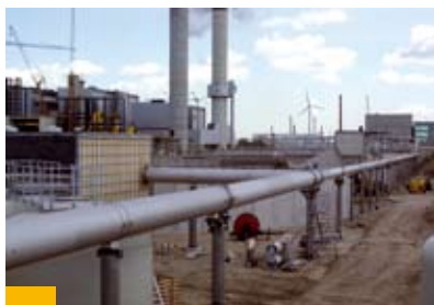
True to our motto "All from a single source" – vessels, pipes and assembly
