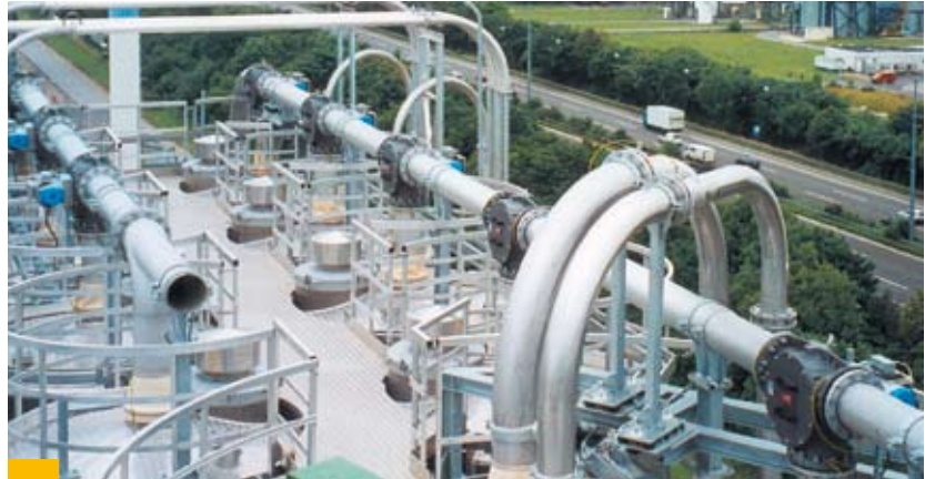
III. 6: Installation of piping systems, elbows, flanges and railings in stainless steel at a chemical plant
