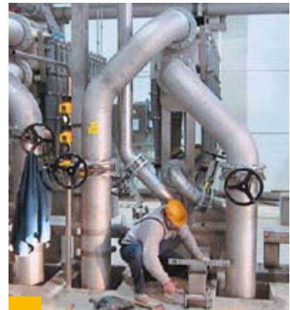
The professional maintenance of a plant is crucially important for its lifetime
