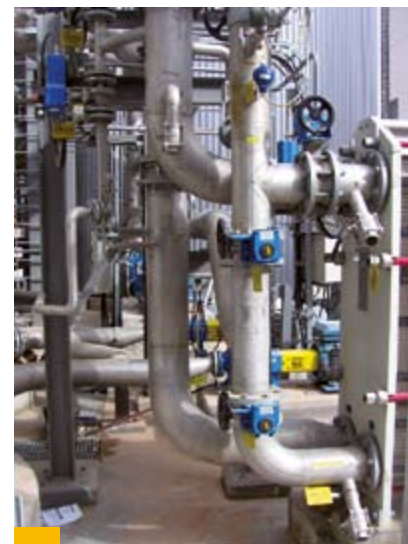
A high degree of prefabrication reduces the need for construction site staff
