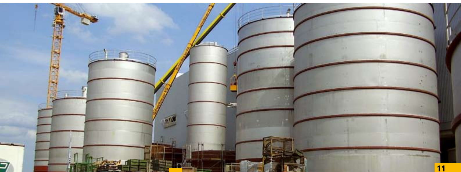
Vessels for the paper mill in Plattling
